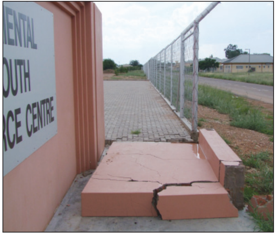
This wall has already fallen, barely two years after it was built. All photos by Levi Upula.
